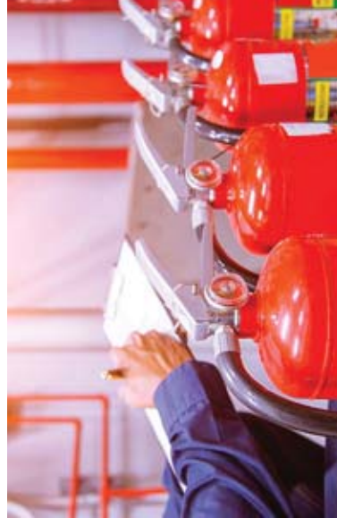
Specialist Fire Suppression System
