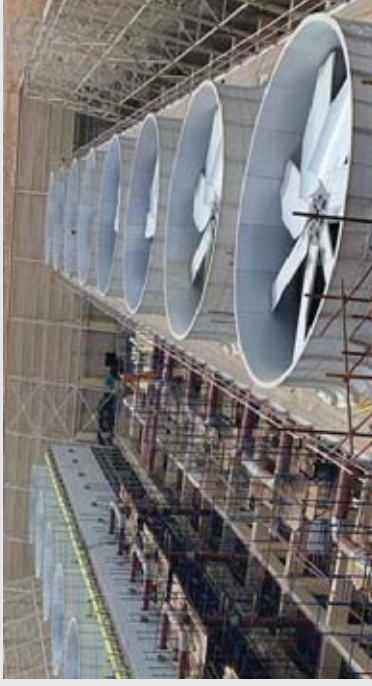
District Cooling Plants
