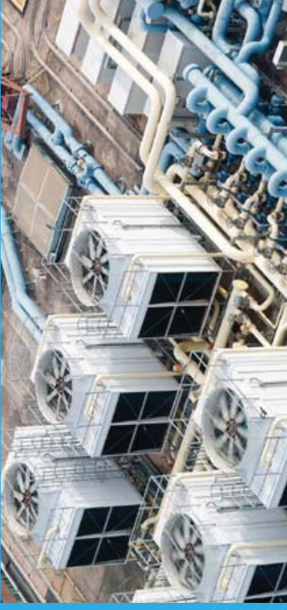
Heating Ventilation and Air-conditioning Cooling (HVAC)
