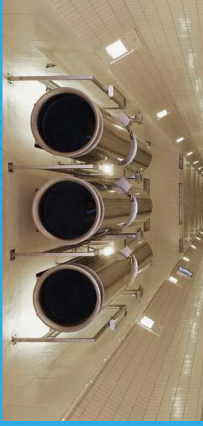
Tunnel Ventilation Services
